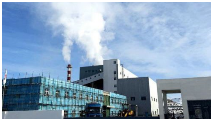
Figure 1. Toson Thermal Power Plant
