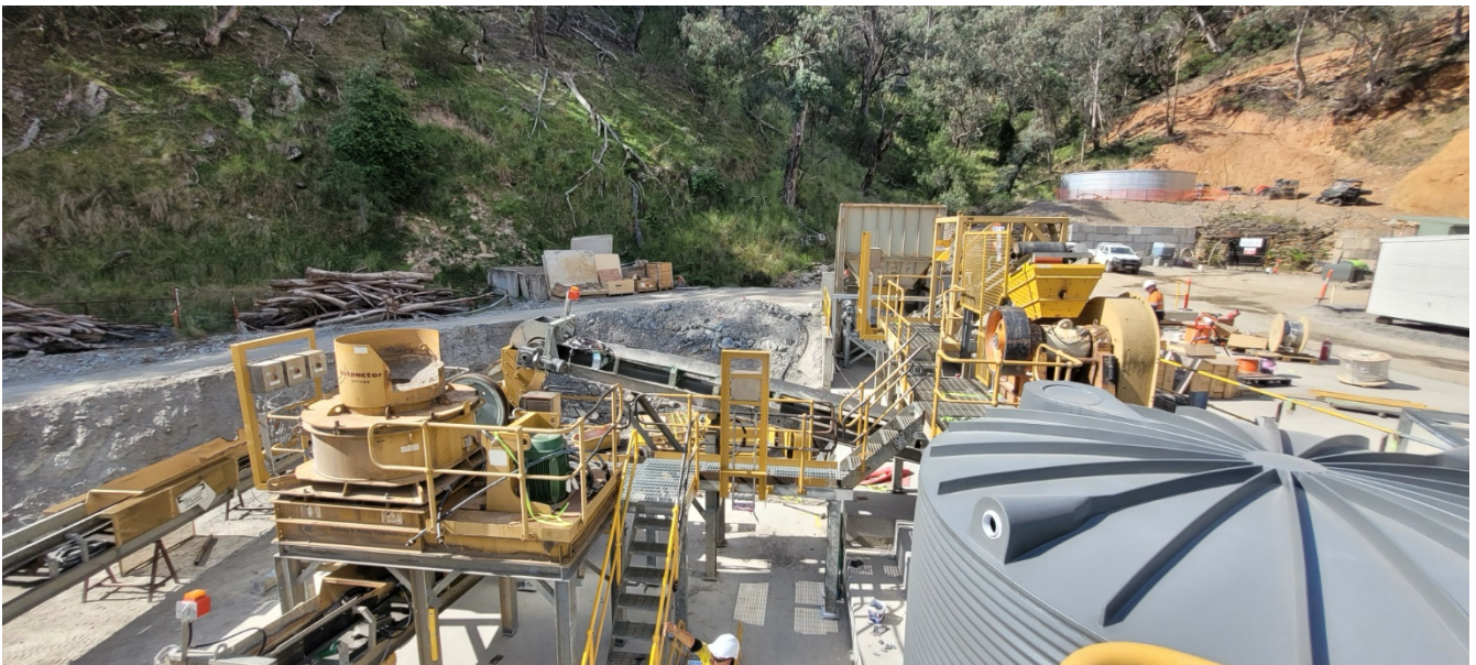
Figure 3 View over the Primary and secondary crusher
