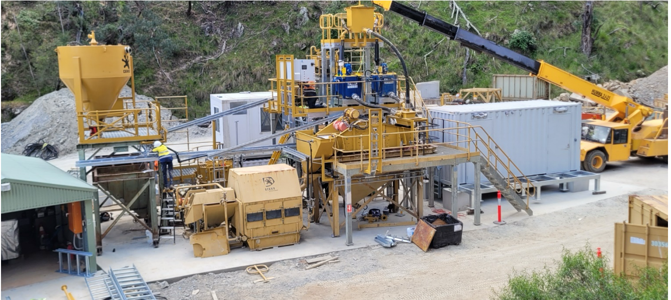
Figure 2 View of the installed plant from Gravity concentrator side
