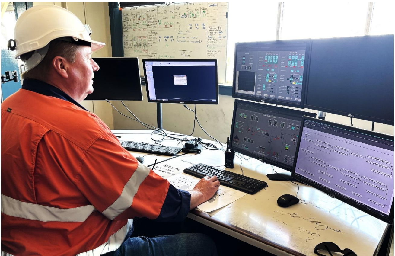
Figure 4: Process plant control and analysis systems upgrade.
