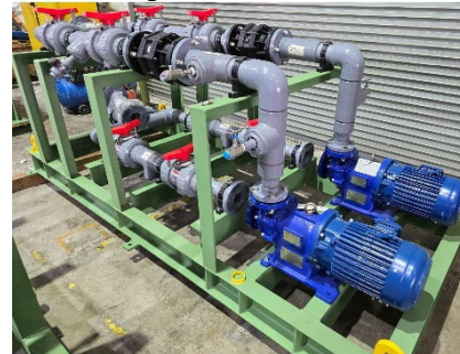
Regen Liquor Transfer Pumps Skid
