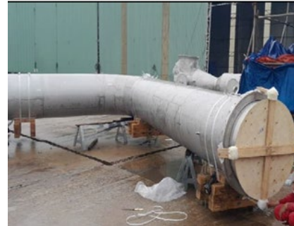
Main Ducting to Venturi Scrubber
