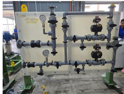
Filtrate Receiver to Storage Tank Piping
