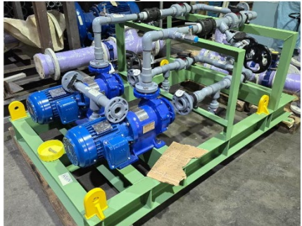
Filtrate Return Pumps Skid
