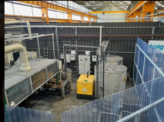
Part of Talnode®-R Pilot Plant
