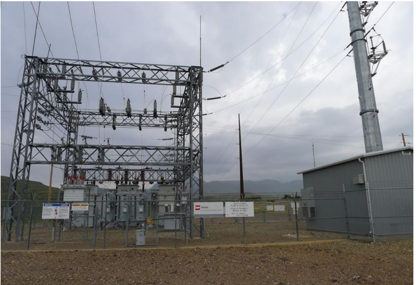
Figure 5: Shafter Mine and Processing Substation.
