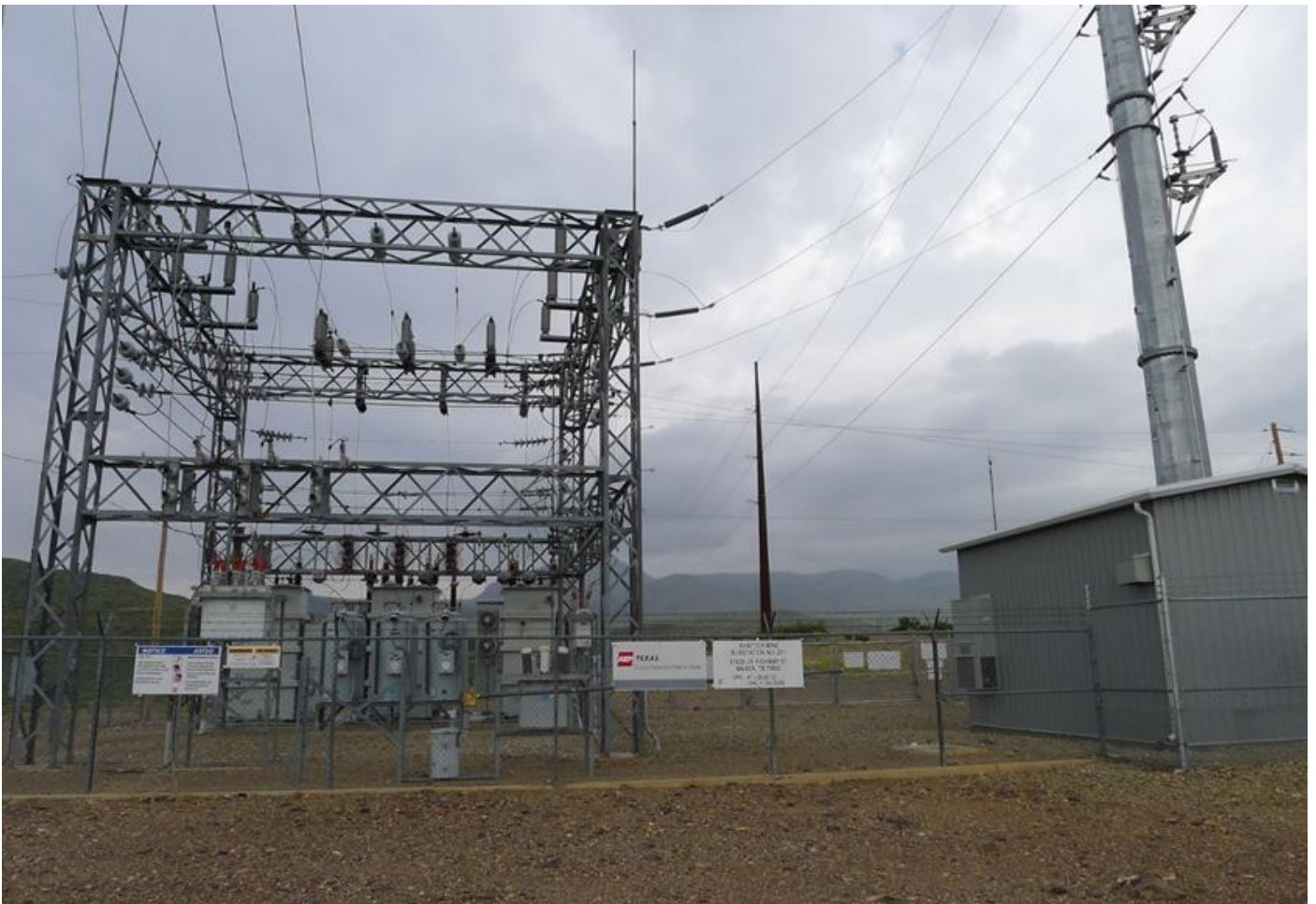
Figure 7: Shafter Mine and Processing Substation.
