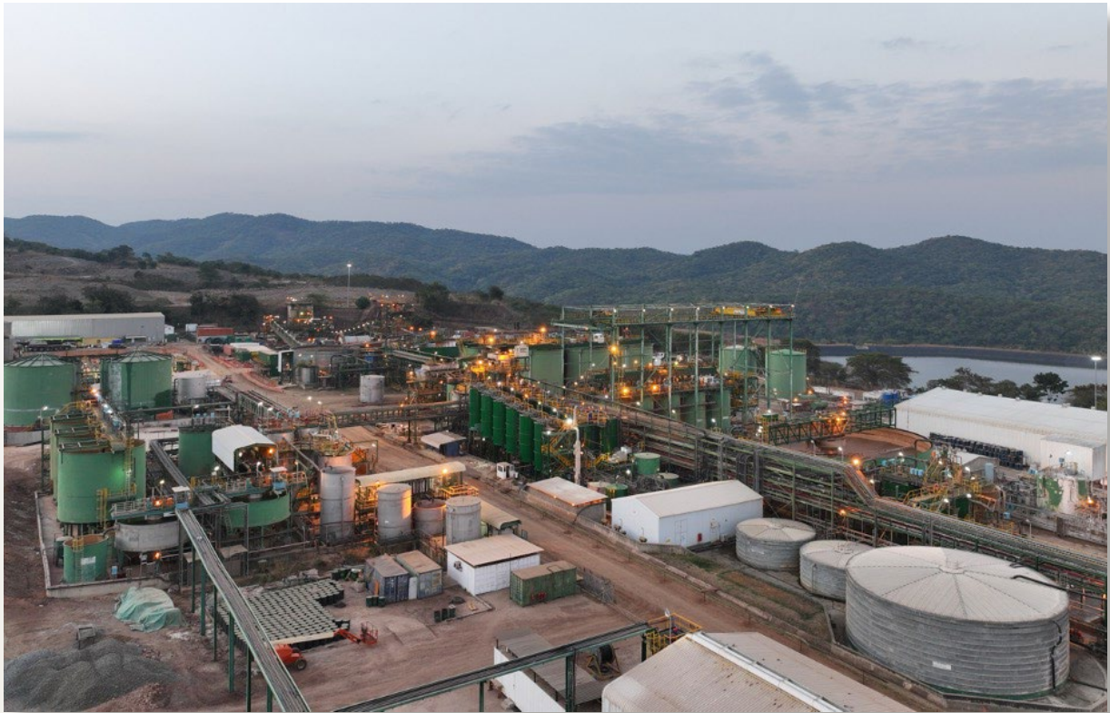
Figure 2: Kayelekera process plant (back end) during commissioning
