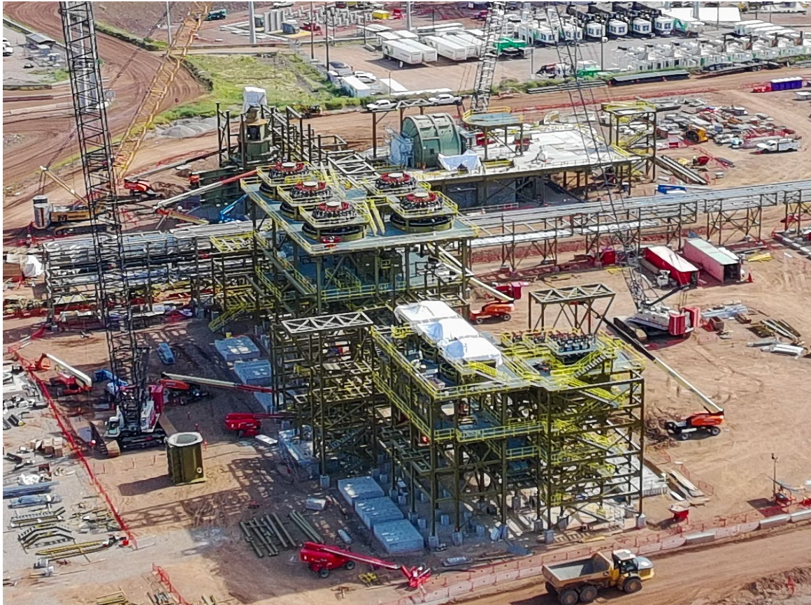
Flotation circuit (looking north)
