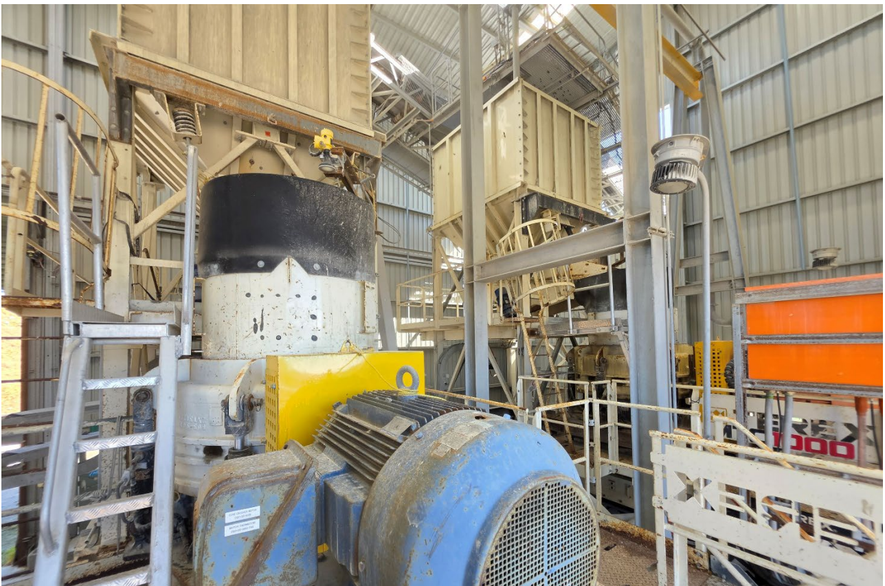
Figure 3: Secondary & tertiary crushers located within the enclosed crushing facility
