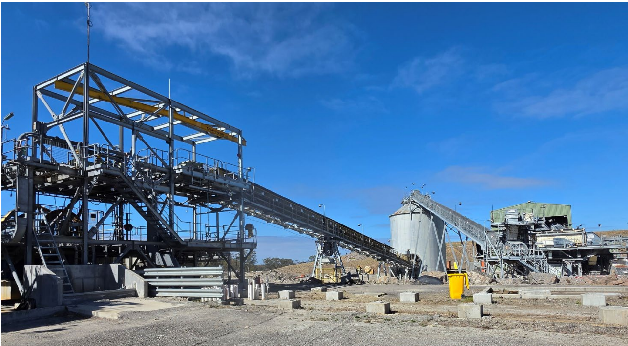
Figure 1: The acquired crushing and processing infrastructure, including mill structure, conveyors & triple-deck screening circuit
