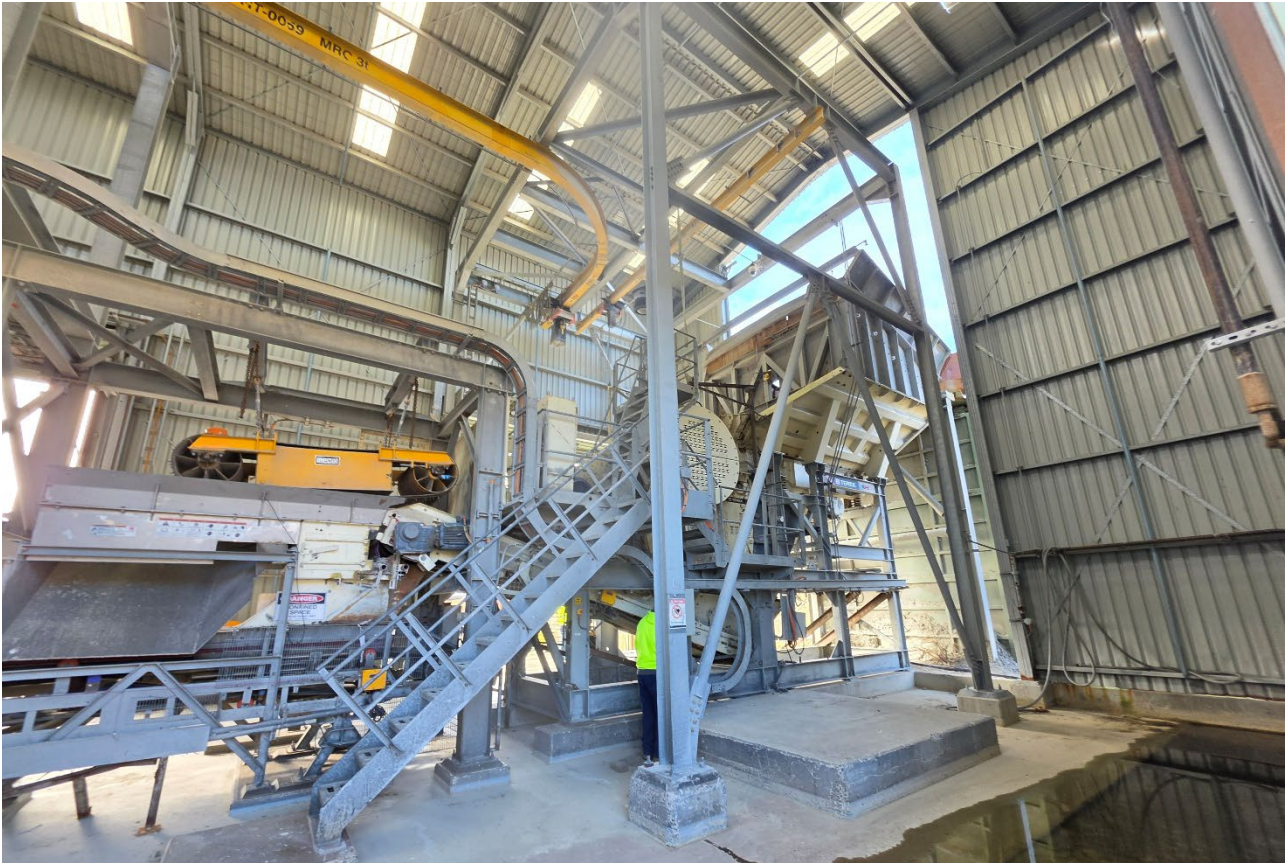
Figure 2: Primary ROM bin and jaw crusher located within the enclosed crushing facility
