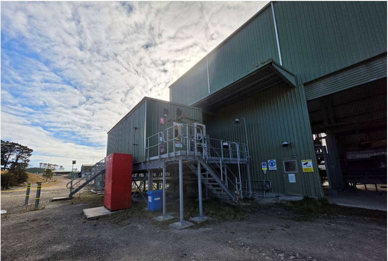
Figure 5: Main crushing motor control centre (MCC) and electrical infrastructure included in the acquisition
