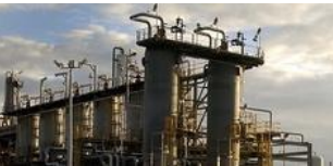
Longford Gas Plant
