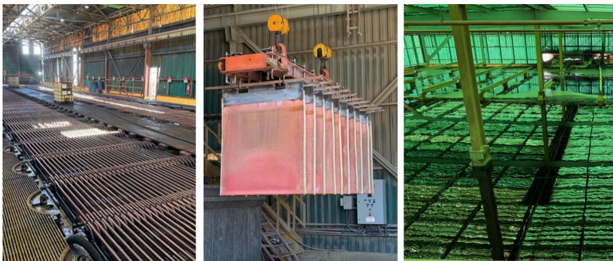
Figure 3. Electrowinning and solvent extraction plants.
