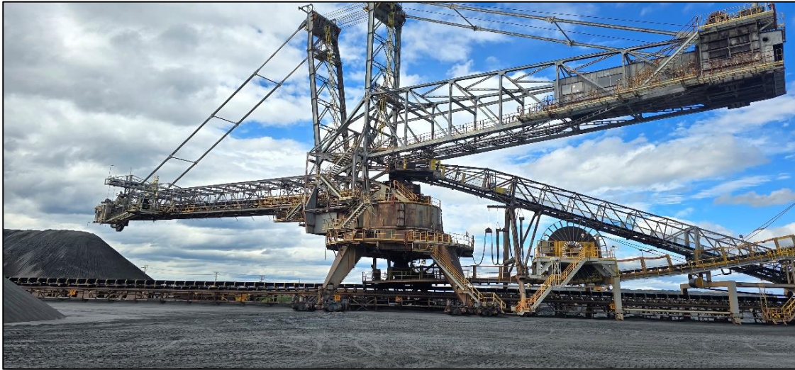
Figure 12: Iron Ore Stacker
