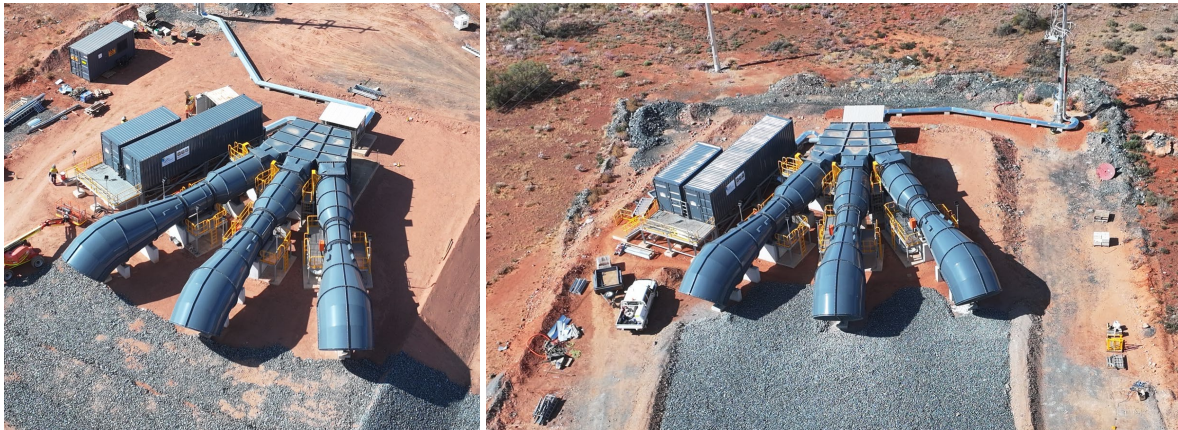
Figure 2: Two major ventilation installations commissioned in September 2024.
