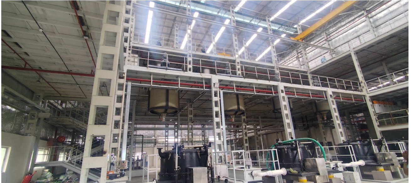
Figure 3 – key components of our plant at PGT
