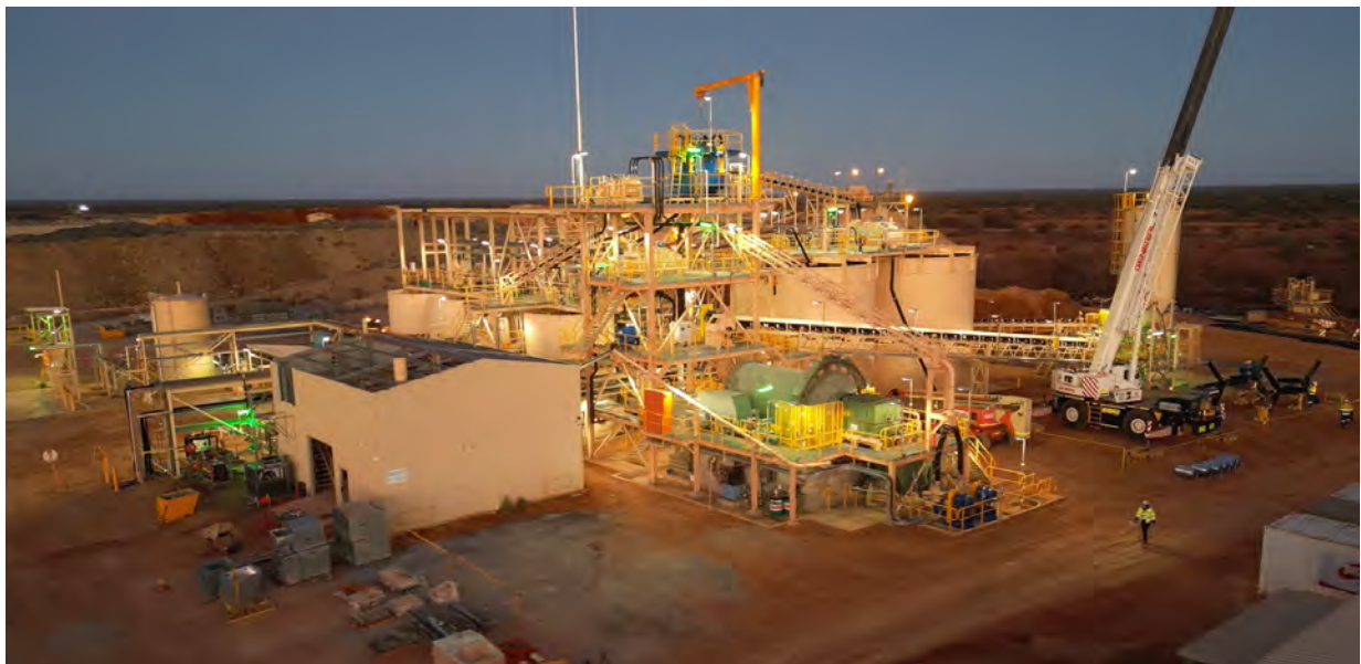
Figure 4: Process plant energised for commissioning.
