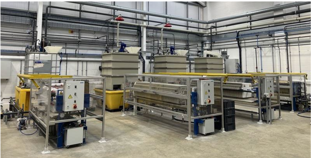
Figure 8: Digestion processes and associated filter presses.
