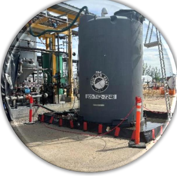
Water treatment plant at Vidalia
