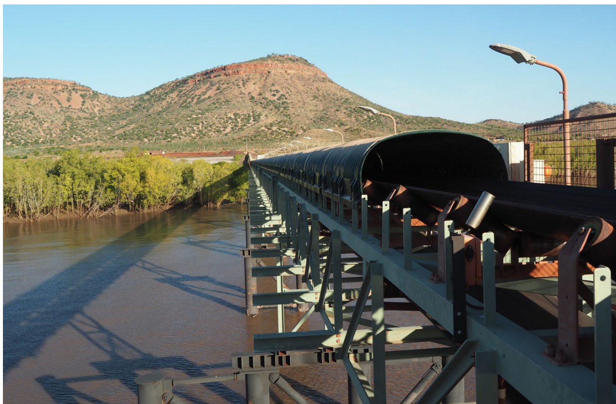
Figure 1: Bulk Loading Facility at Wyndham Port
