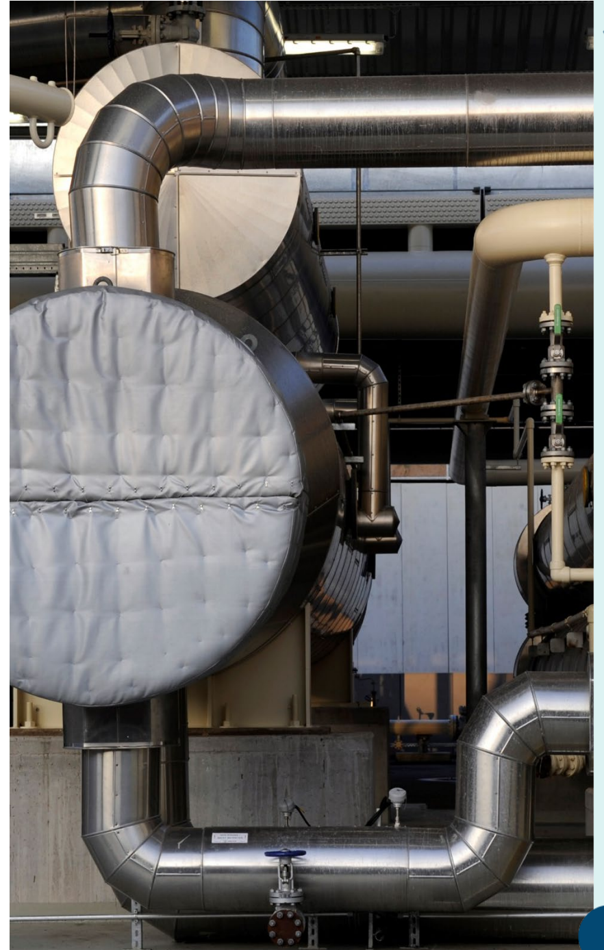
Vulcan's Insheim Geothermal Power Plant
