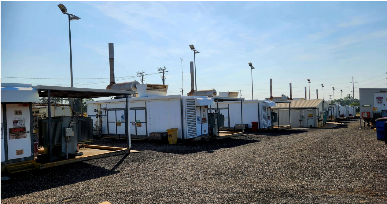
Image: Moranbah Power Station
