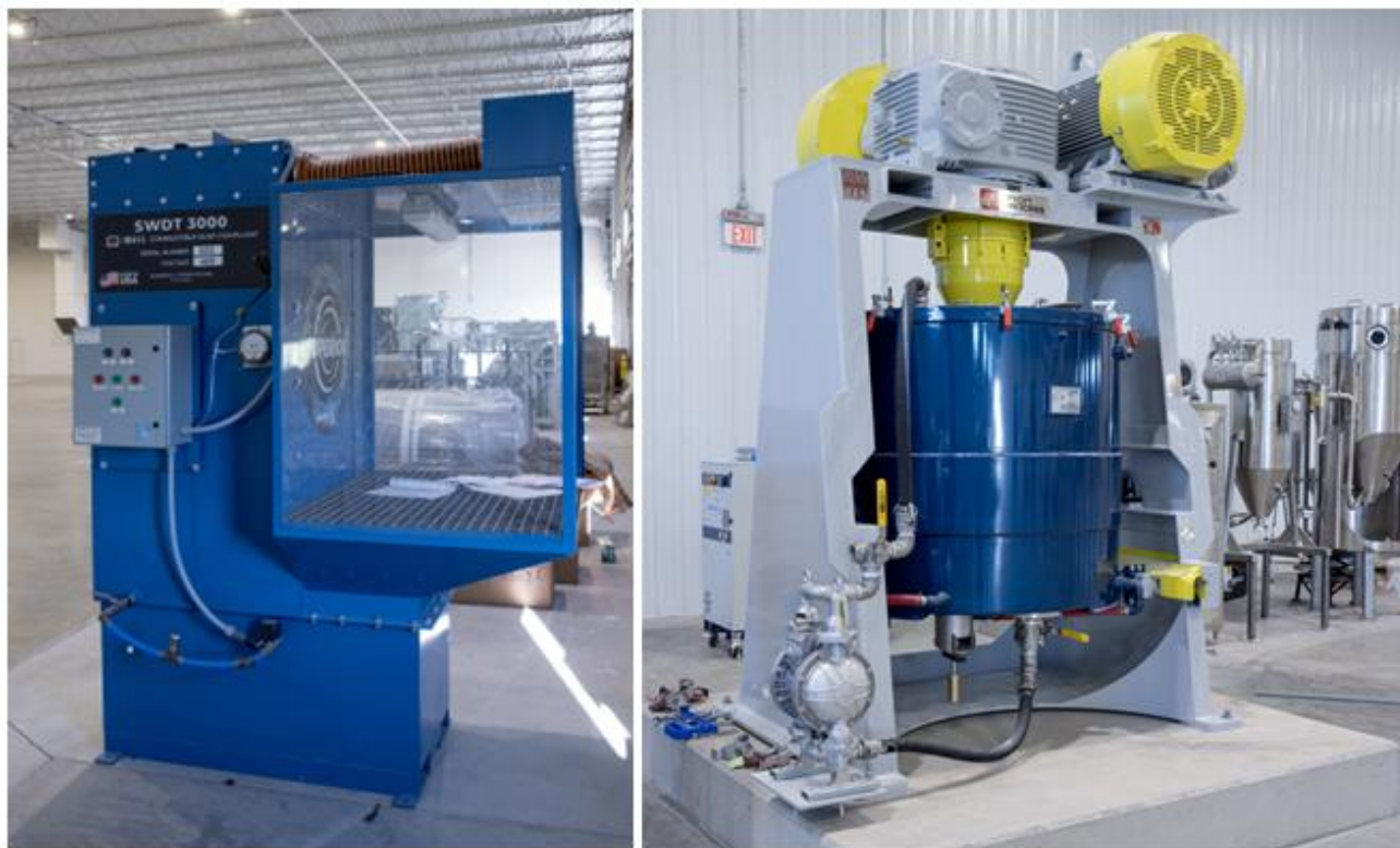
Figure 2: Ancillary operations equipment installed at the Titanium Production Facility
