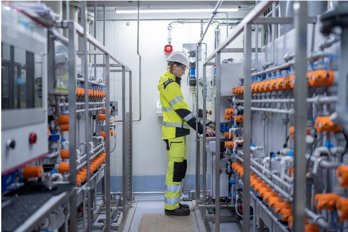
Figure 13 Reverse osmosis unit at Vulcan's upstream LEOP
