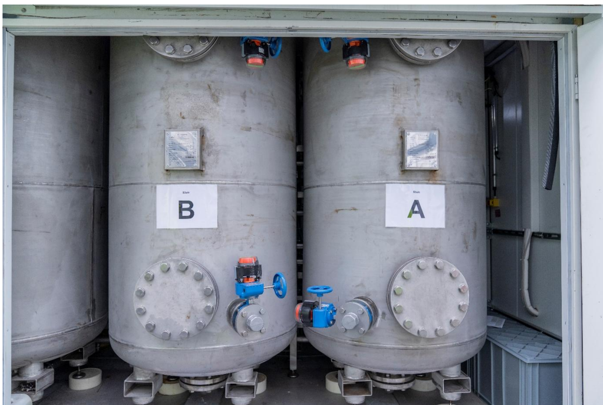
Figure 1 Vulcan's A-DLE unit at the upstream LEOP in Landau, Germany
