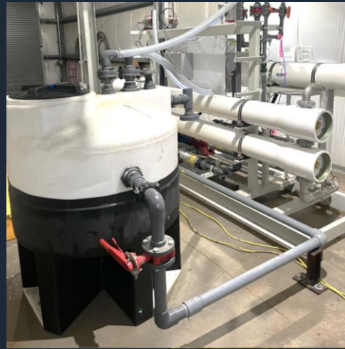
Reverse osmosis plant at Vidalia
