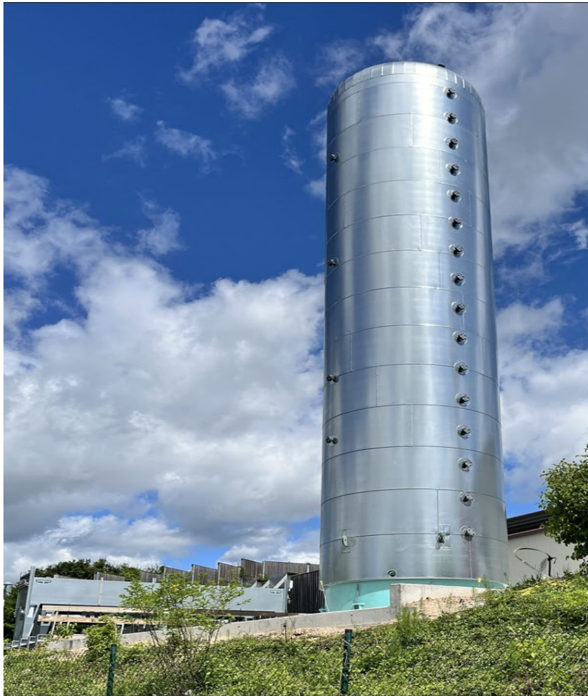
Figure 2 Thermal energy storage facility on site at Vulcan's Natürlich Insheim geothermal renewable energy plant for the GEOSMART project.
