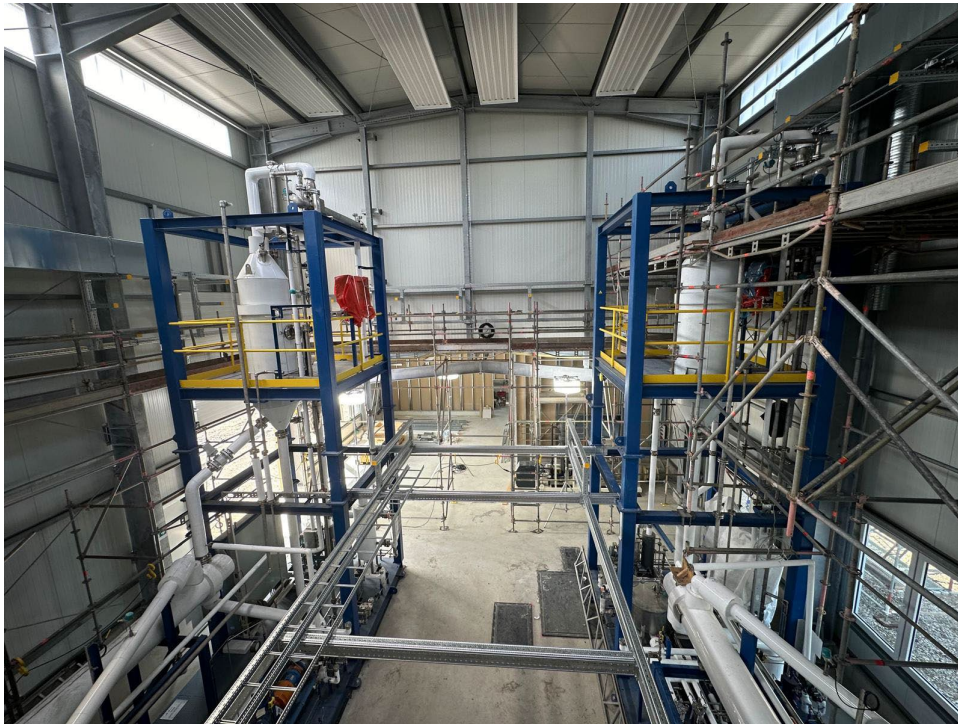
Figure 4 Inside Vulcan's CLEOP, showing the two newly-installed crystallisers.
