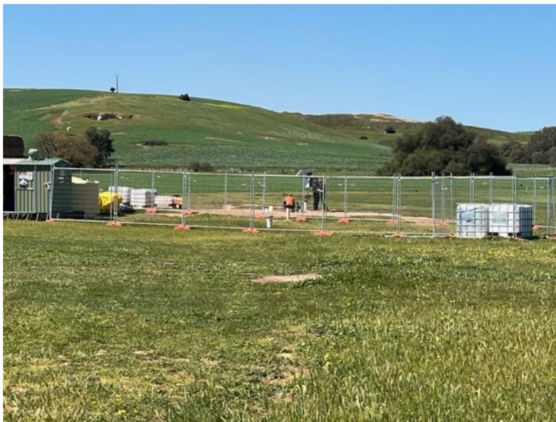
Photo 1: Well house and bores for push/pull tests, Kapunda
