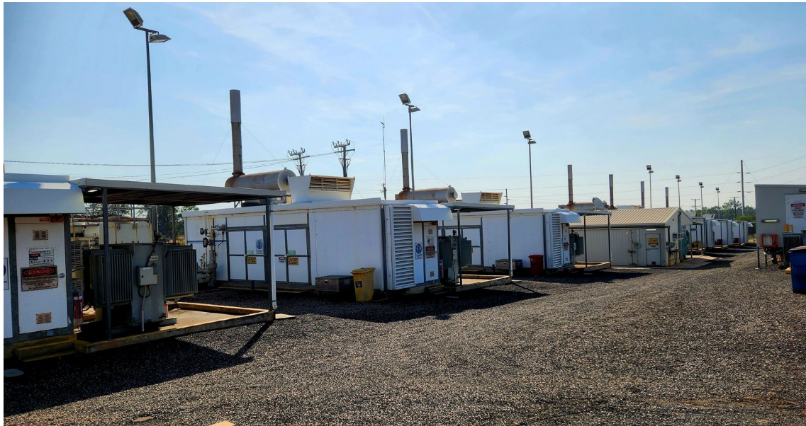
Image: Moranbah Power Station
