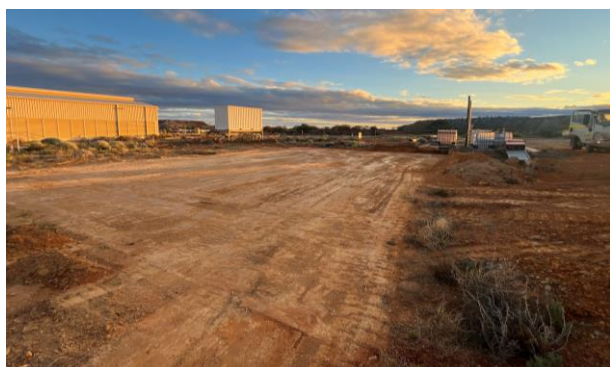
Figure 3: New fuel farm pad (foreground), power station (background), July 2024.
