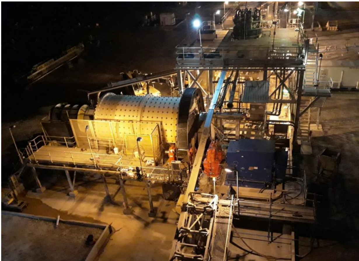
Figure A16: Existing 1800kW Ball Mill
