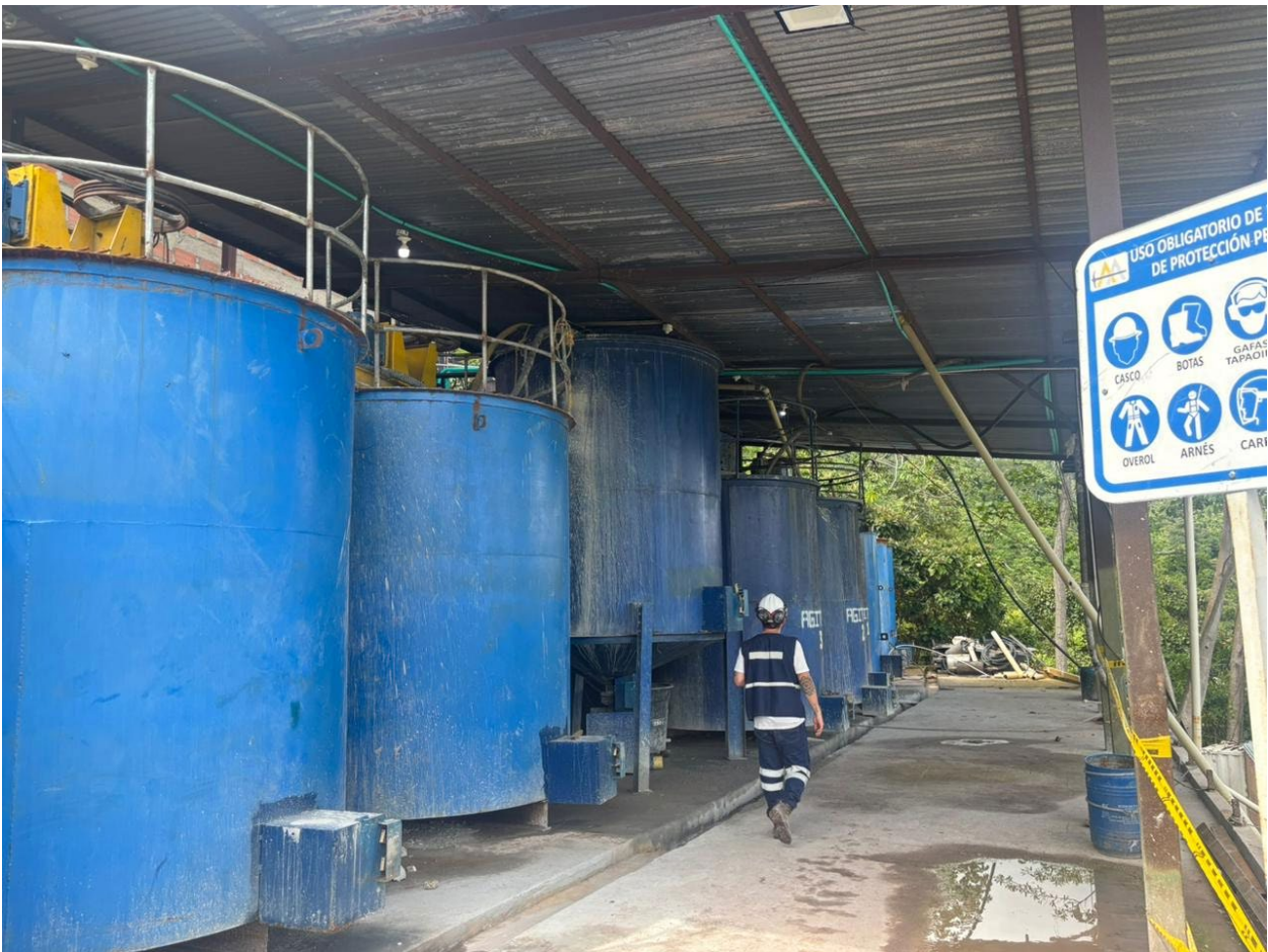
Photograph 1: Agitation tanks, Santa Barbara Processing Plant
