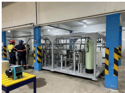
Figure 8 – Water Treatment skid installed
