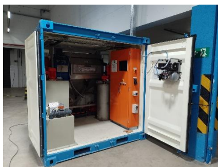
Figure 9 – Filtration unit installed
