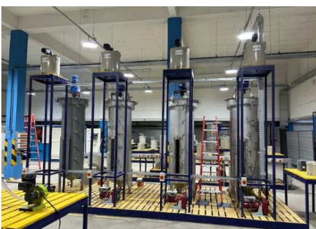
Figure 5 – CCD circuit all plumbed up
