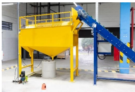
Figure 3 - Ore feed conveyor and scrubber
