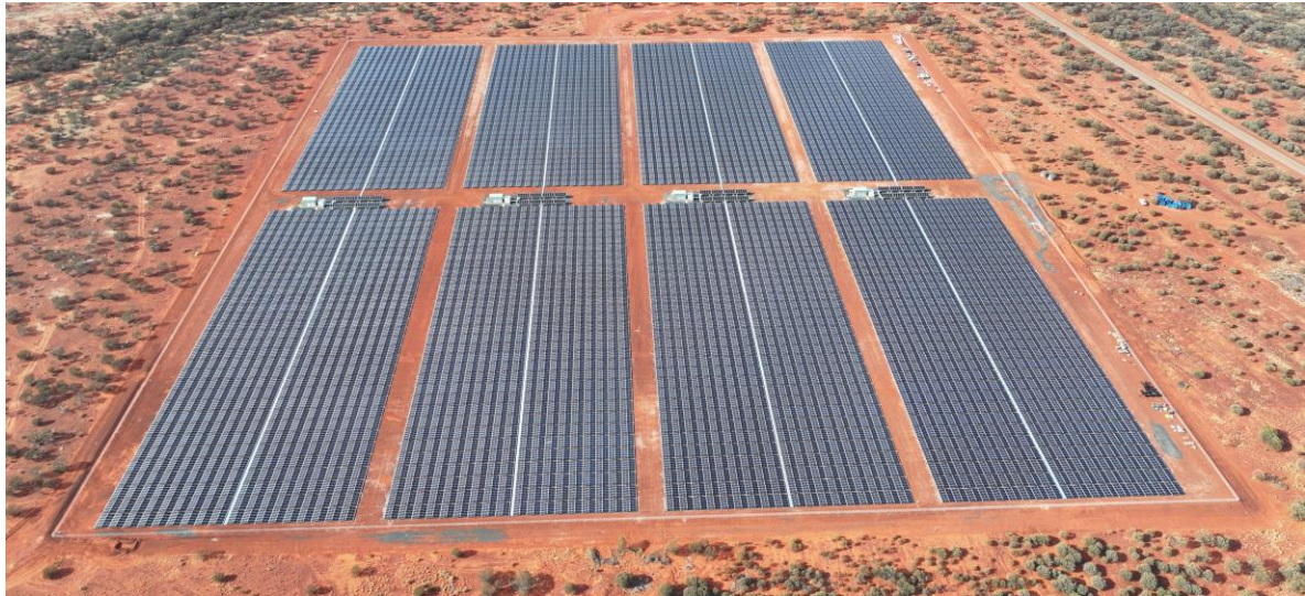
Solar – 27MW solar installation
