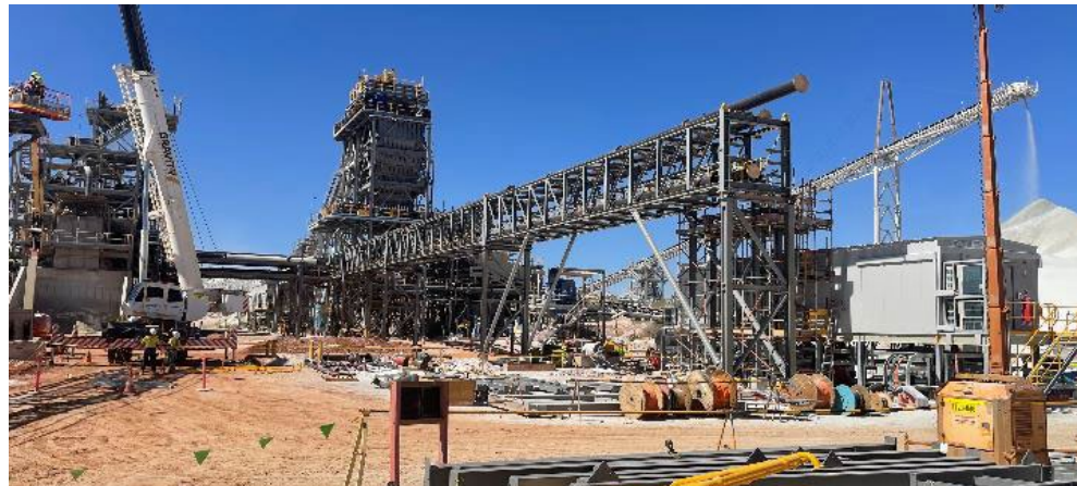
Primary rejection infrastructure
