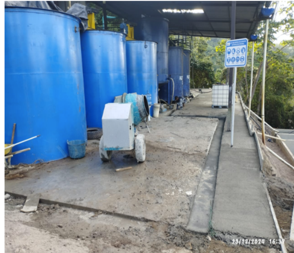
Expanded Agitation section, Santa Barbara processing plant
