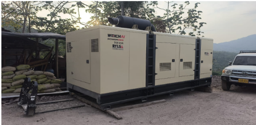
A second standby generator will be added in the coming months
