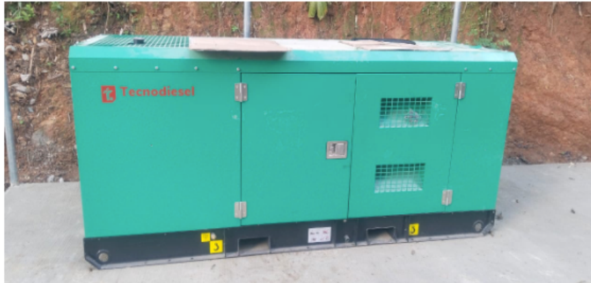
Underground mine power now provided by two 75kva diesel generators
