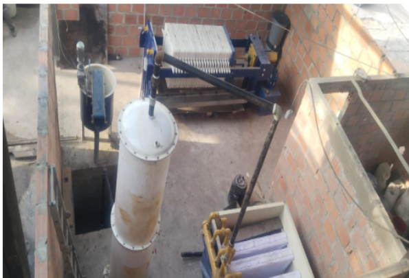
New Merrill Crowe precipitation system, Santa Barbara processing plant
