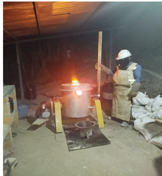
New gold room electric furnace, Santa Barbara processing plant
