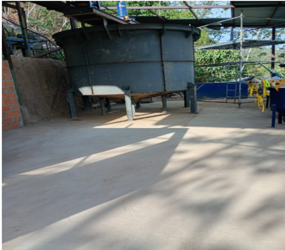
New thickener, Santa Barbara processing plant
